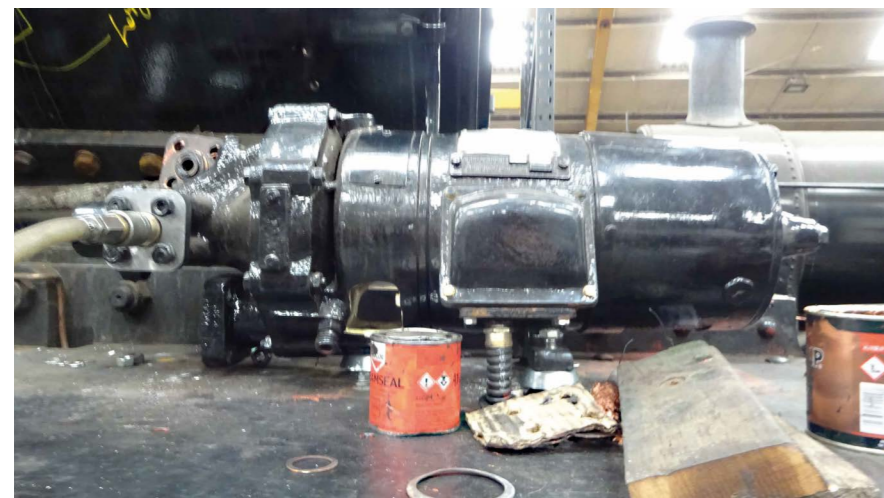
Above: Old turbogen under test with air.
