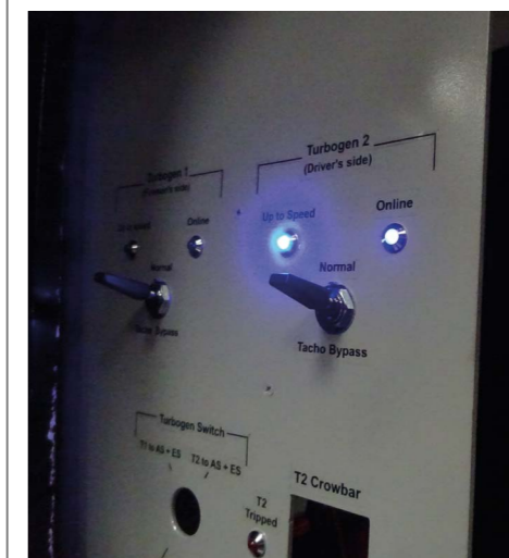
New turbogen up to speed and delivering power to the electrical system.
