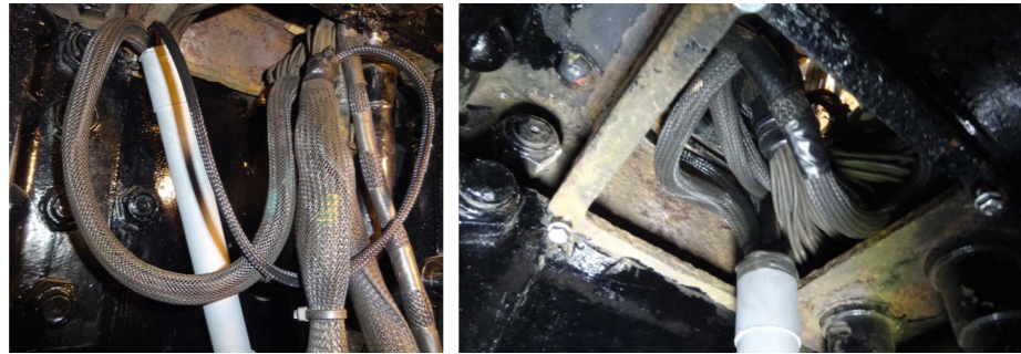
Above left: Loom connected in to harnesses and protected with braided sleeving and right, AS conduit box with all harnesses in place into the cab above.
