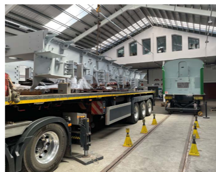
Frames delivered to DLW in primer, and positioned in front of the tender tank and wheels.
