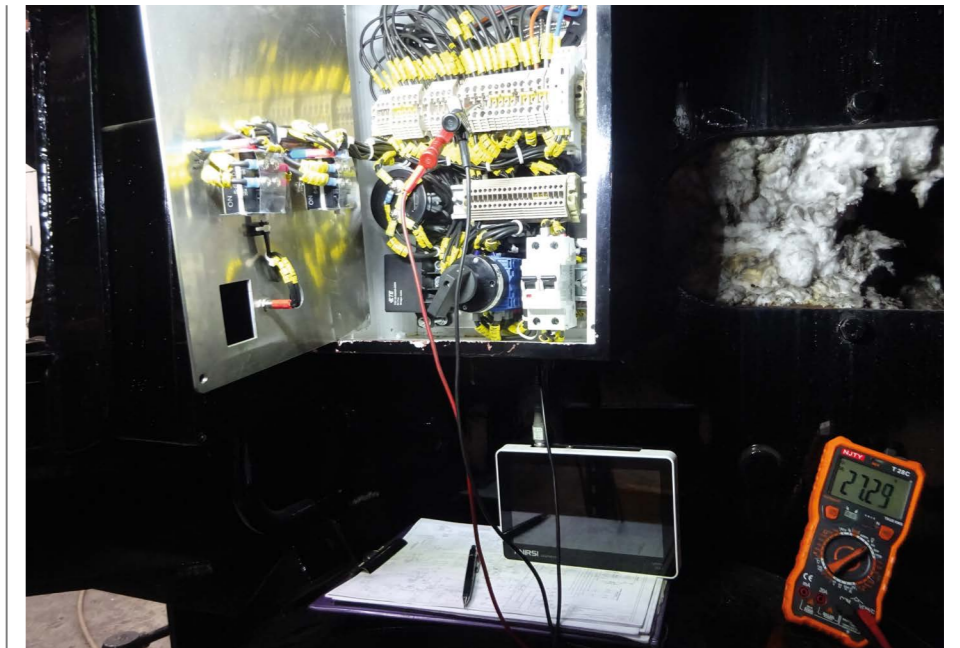
New turbogen generating for the first time.
