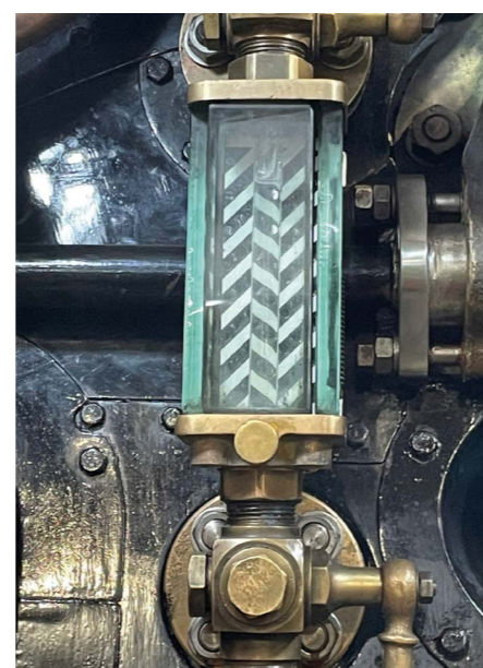
Gauge glass showing the boiler topped up ready for steaming.
