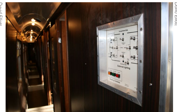
The Lighting mimic panel
